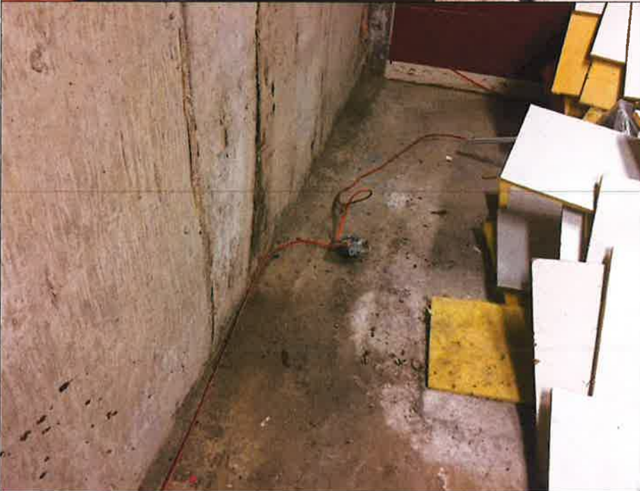
Photo 14: Note signs of water ingress at wide crack in west foundation wall
