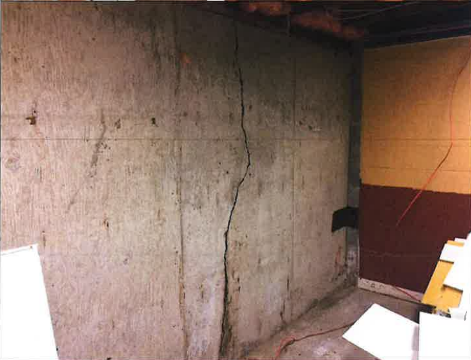
Photo 12: Typical foundation wall - Note wide vertical crack
