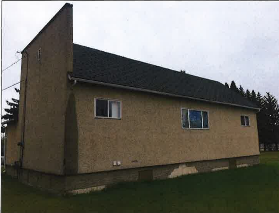
Photo 3: West Elevation – Note missing sections of downspout and water damage to stucco
