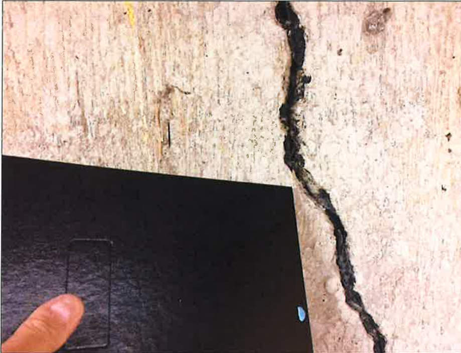
Photo 13: Wide vertical crack in west foundation wall – Note previous attempt to seal crack
